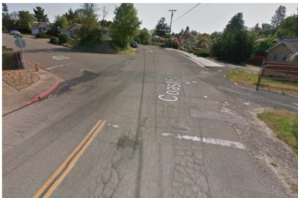
Figure 121: The intersection of Coast Street and Mill Street is lacking ADA accessible curb ramps at three corners (Source: Google Street View)
