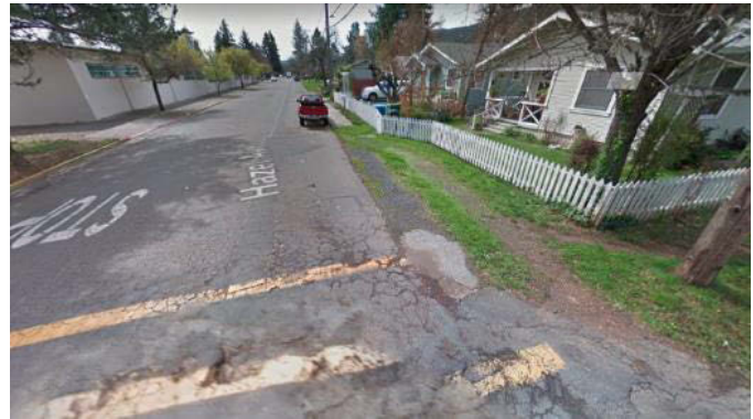
Figure 58: Sidewalk gap along Hazel Avenue (Source: Google Street View)
