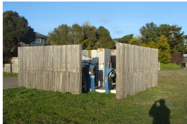
480V service adjacent to parking
