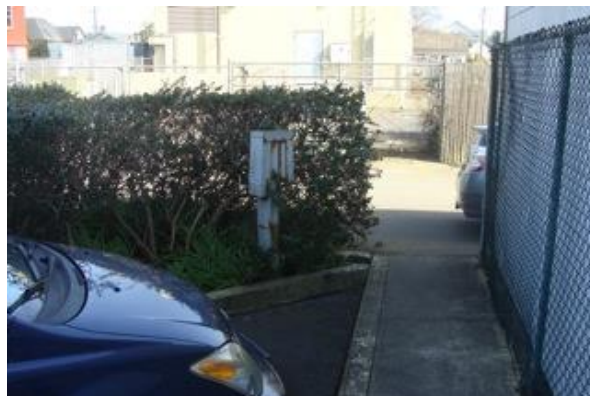
Dismantled EV charger in City parking lot
