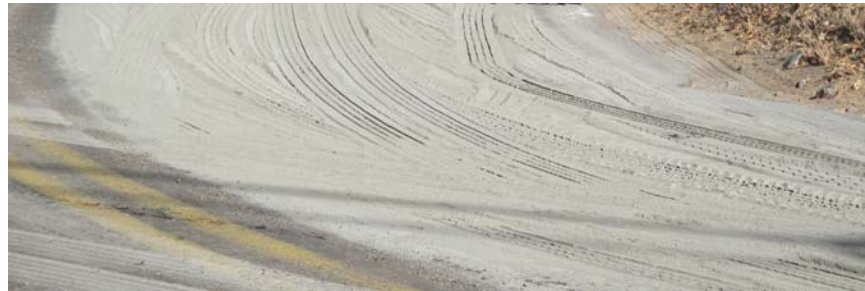
Spread some cement out to grind into old road surface & Aggregate Base Rock (AB)
